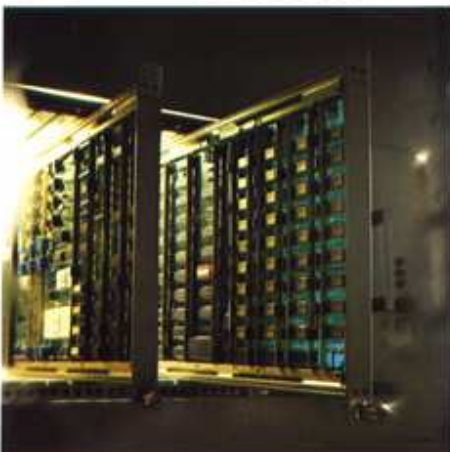
CR80 Crate with module pulled out
