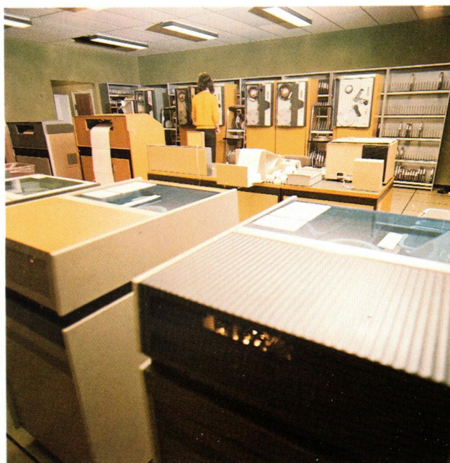
RC 4000 anlæg i RC's servicecenter i København. RC 4000 computer installation at RC's service bureau in Copenhagen.
